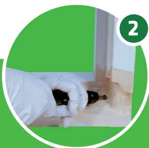
Remove all decay
