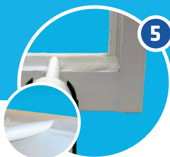
5 Cut the nozzle to form the glazing profile and apply DRY SEAL™
