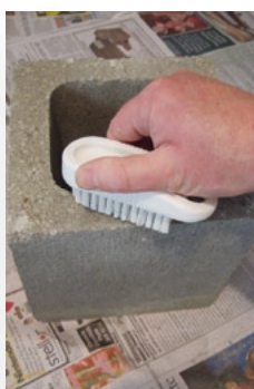
Step two Brush the blocks with a stiff bristled brush to remove any dust and loose concrete material.
