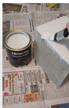
Step four Prime the blocks with one coat of Resene Concrete Primer and allow to dry for two hours.
