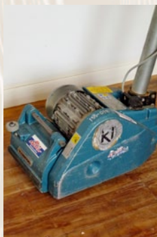
Step five Again, using appropriate floor sanding equipment and wearing recommended protective clothing, carefully sand the remainder of the floor, sanding in the direction of the grain.
