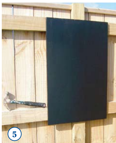
5 ATTACH the ply panel to the fence with 40mm galvanised nails. Touch up the nail heads and any marks with a coat of Resene Nero.
