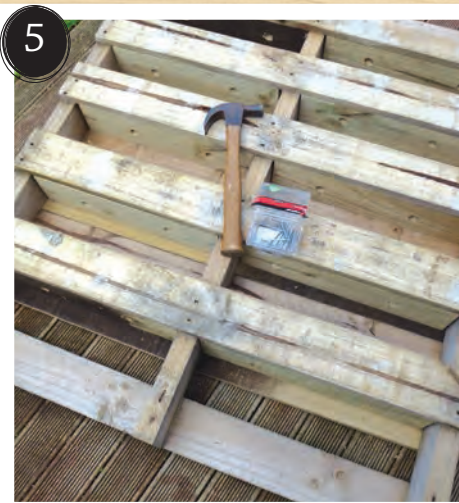
Attach the bases into position, as shown, fixing from the front with 50mm nails.
