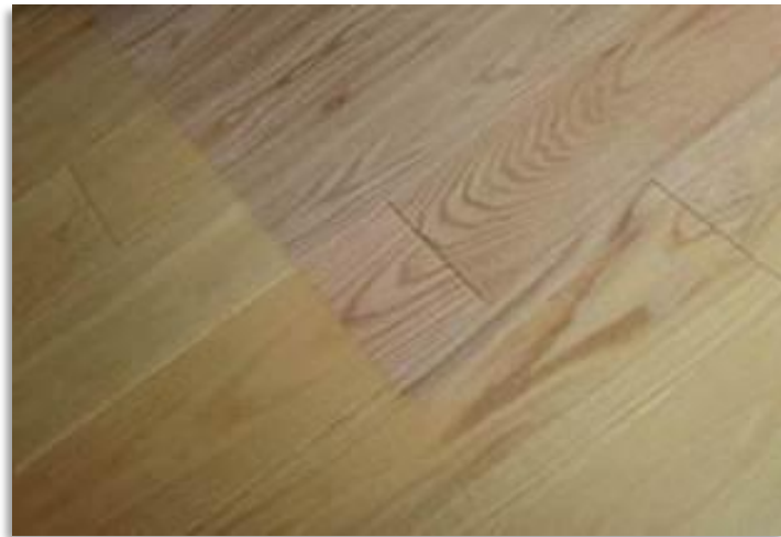
Flooring that has had a carpet rug moved
